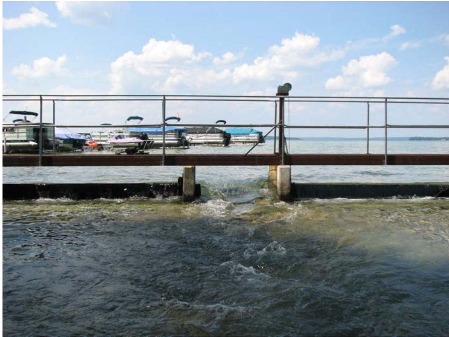
Unregulated span viewed from downstream face. Note the rubber restrictor on the left side of the opening.
