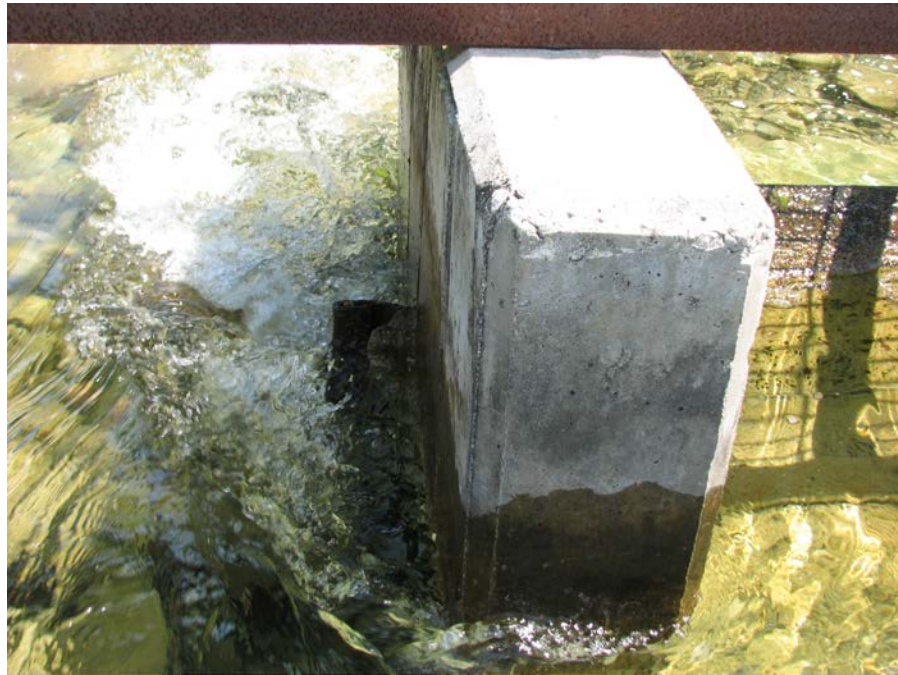
4-inch rubber restrictor in center open span.
