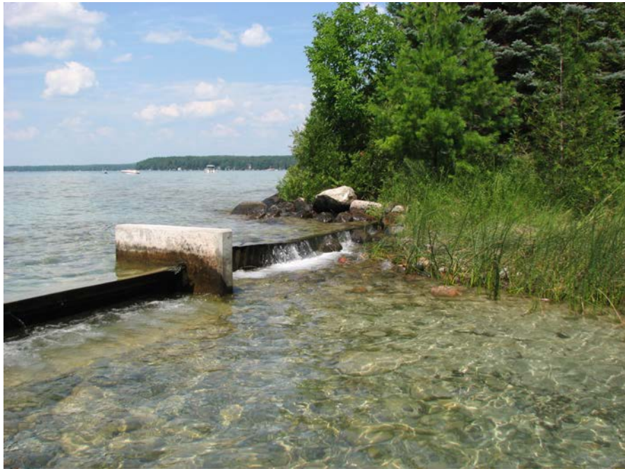
Downstream face of the sheet pile weir at the northern end of the Higgins Lake LCS.
