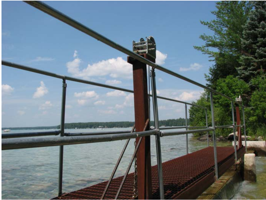
Flop gate hoists on downstream railing of Higgins Lake LCS.
