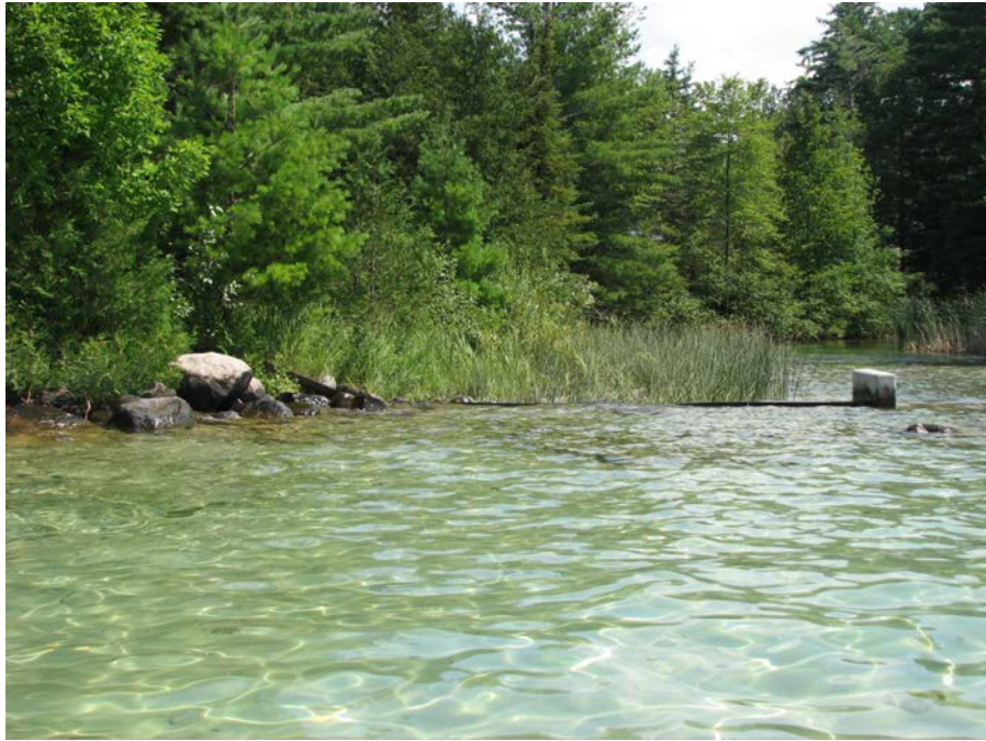
Upstream face of the sheet pile weir at the northern end of the Higgins Lake LCS.
